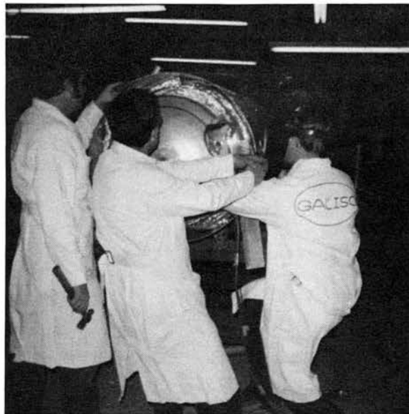
Mogens Friedlow (L) looks on as Galiso founder and the dewar's designer, Carl Grenche, (center) supports the inner head of the dewar with a piece of lumber as an unidentified technician welds the unit closed.
